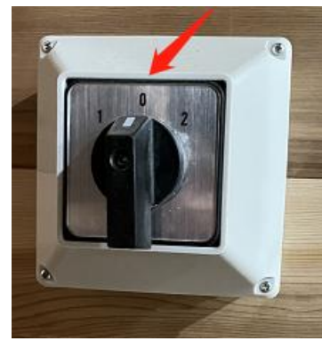
Power turned OFF
