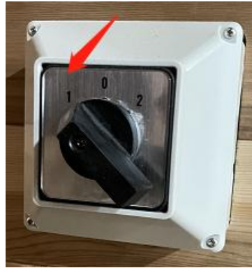
Power to stove heater
