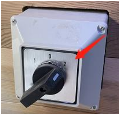
Power to Infrared heaters
