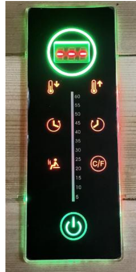
Sauna's Control Panel is ON (control panel illuminated)
