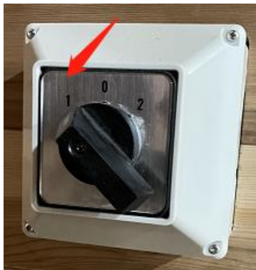
Power to stove heater
