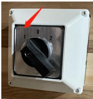
Power to stove heater
