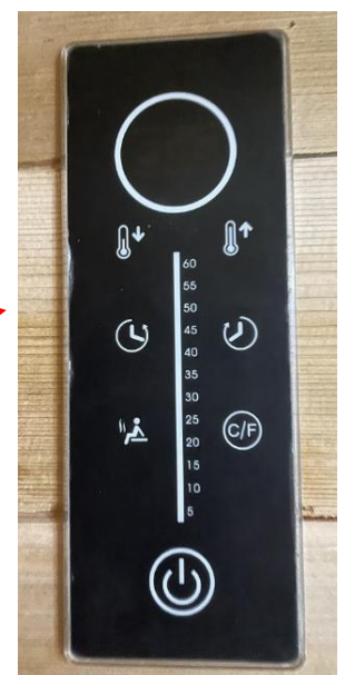
Sauna Control Panel has no Illumination
