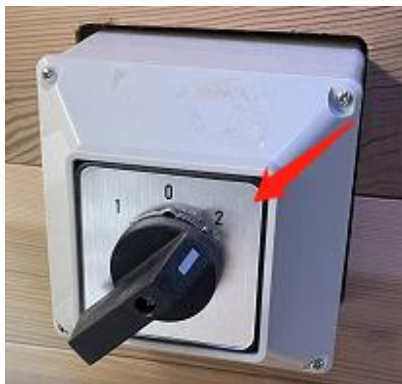
Power to Infrared heaters
