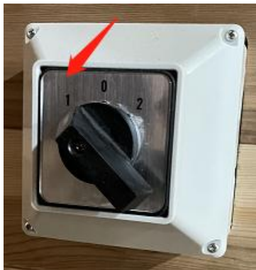
Power to stove heater
