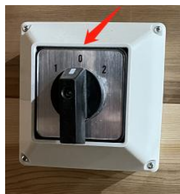
Power turned OFF
