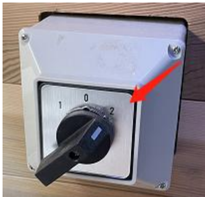
Power to Infrared heaters
