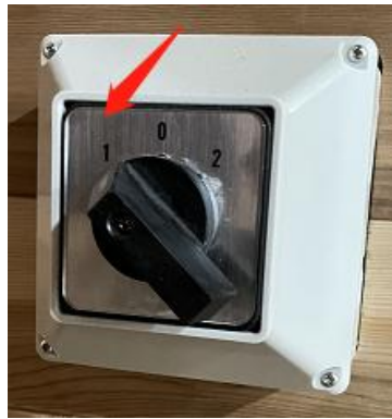
Power to stove heater
