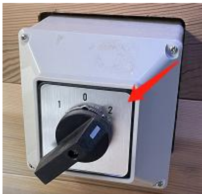
Power to Infrared heaters
