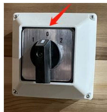
Power turned OFF
