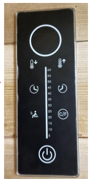
Sauna Control Panel has no Illumination
