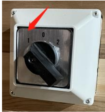
Power to stove heater
