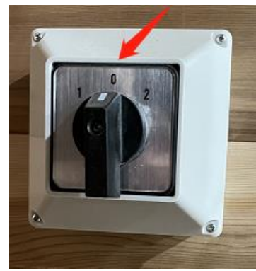
Power turned OFF
