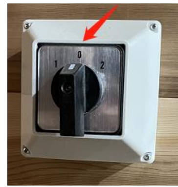
Power turned OFF
