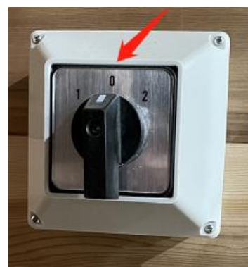
Power turned OFF
